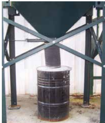
A storage drum prevents dust from backing up in the hopper and creating an explosion hazard.
