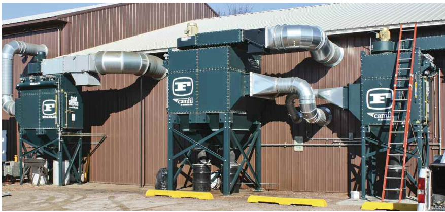
From left to right, seen outside the Fast trio of adjoining buildings: a Farr Gold Series GS8 dust collector installed in 2009 to tackle weld fumes; a GS16 installed in 2011 that captures laser-cutting dust and fumes; and a GS6 installed in 2012, also for laser-cutting fumes and dust.
