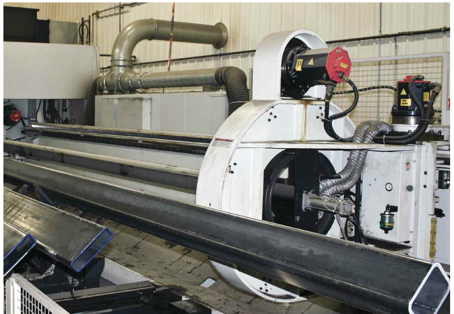
Ducting from Fast Manufacturing's Mazak laser tube-cutting machine leads to a Farr Gold Series GS8 dust collector, located outdoors.
