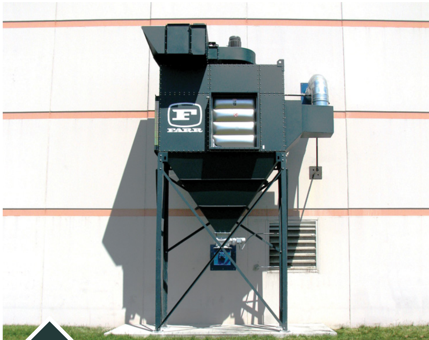
Figure 3. Cartridge dust collector with venting to expel explosion away from building.
