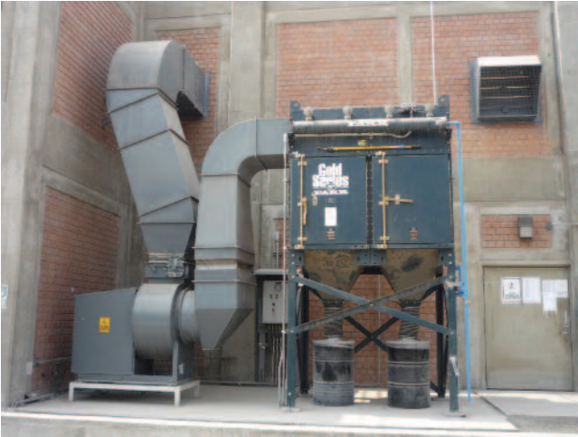
A 16-cartridge dust collector pressurizes and ventilates a compressor room in a power generation plant. Wall louvers allow for air exchange and are calibrated to maintain a specific pressure inside the facility.
