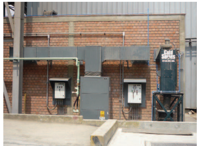
A small cartridge collector is used to pressurize an electrical room. Located in a warm climate, the room has its own backpack-type air conditioning unit for cooling, and the dust collector is sized for 10 percent of the capacity of this unit.
