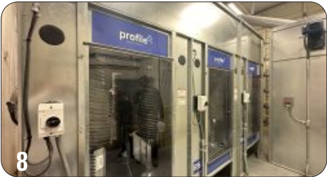
Rotary spirals from Profile Industries were installed in October at the Mid-State Seed production plant in Marshall, MO. The equipment is designed to help produce cleaner seeds, including soybeans. (Profile Industries)
