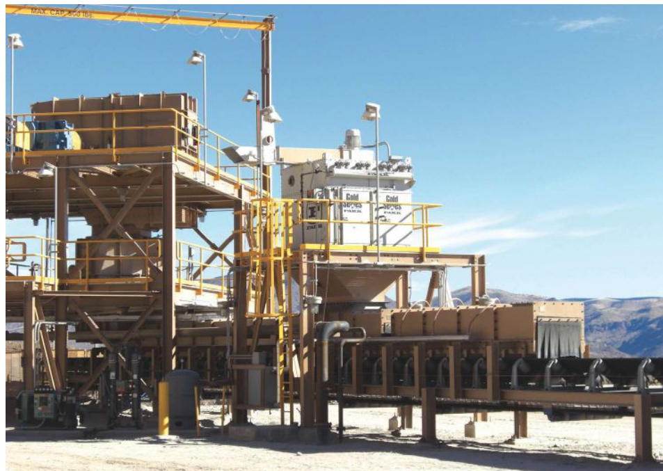
A conveyor transfer combines dust control techniques using containment and a collector along with water sprays.
