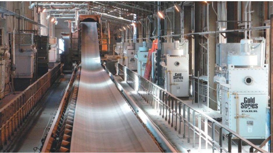
A tripper car installation uses seals, ventilation and collection systems to contain dust.
