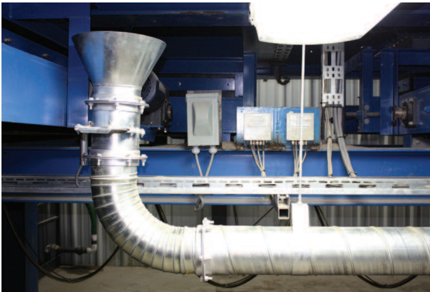
This 6-inch duct pickup under the silos pulls the fugitive silica dust out of the atmosphere and into the dust collector.
