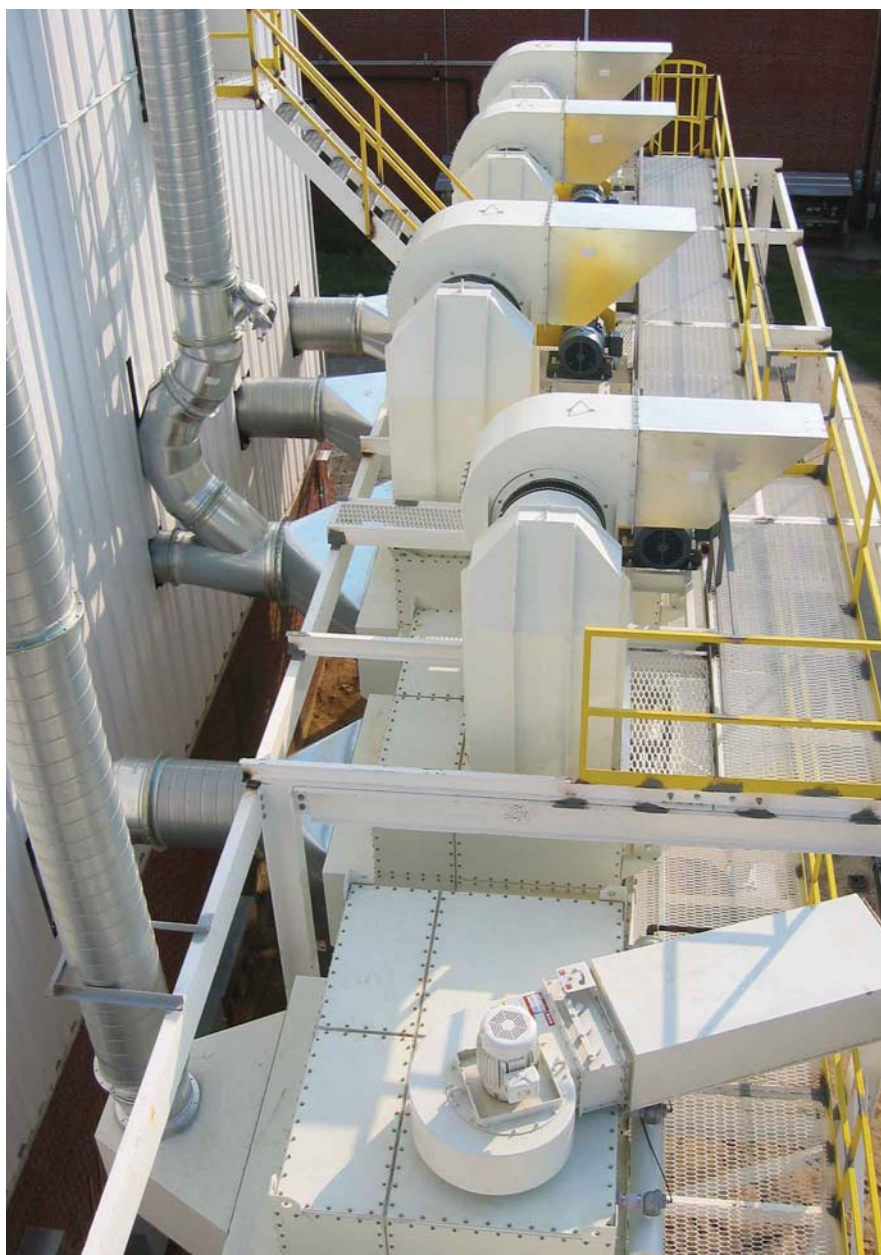
The engineering firm designed and built platforms around the dust collectors and stairways, allowing operators easy access for maintenance checks and filter changes.
