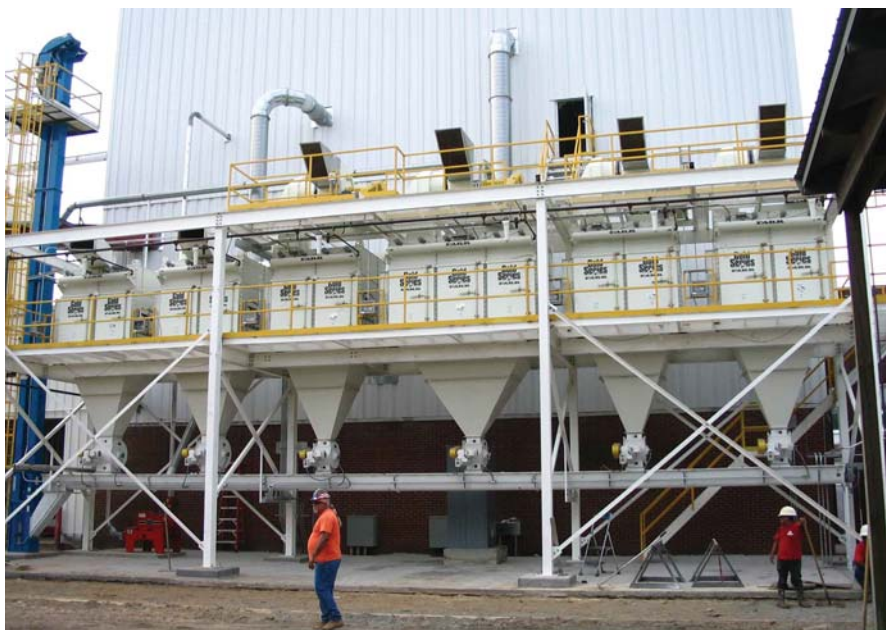
Six dust collectors, which are installed side by side on a custom-built support structure, generate a total airflow of around 90,000 cfm to effectively remove dust from the production facility.
