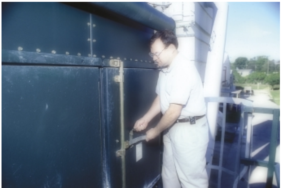
Ricky Criss prepares to open heavy duty access door to the dust collector.
